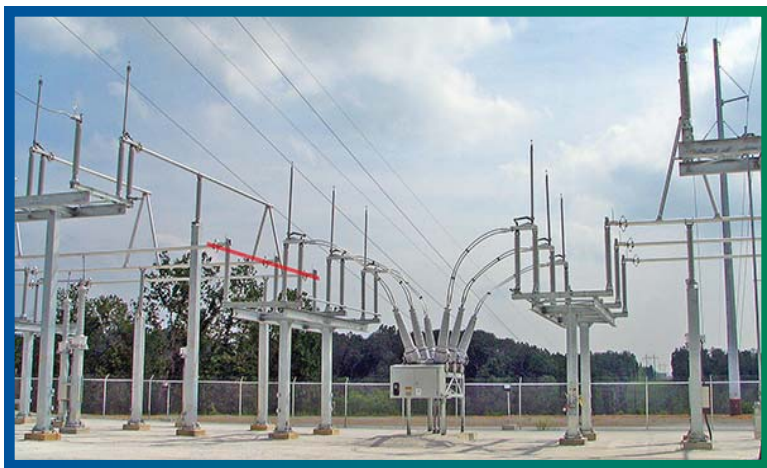
OPEN SWITCHES STAND AT THE READY AS THE HILLTOP INTERCONNECTION NEARS COMPLETION. THE RED LINE SHOWS THE DEMARCATION BETWEEN ENTERGY’S EQUIPMENT (TO THE RIGHT OF THE LINE) AND SOUTHWESTERN’S (TO THE LEFT). SOUTHWESTERN’S BULL SHOALS TO DARDANELLE LINE APPEARS OVERHEAD.
